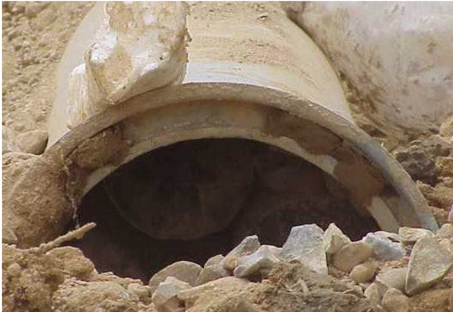
Projectiles inside of a roadside culvert pipe
