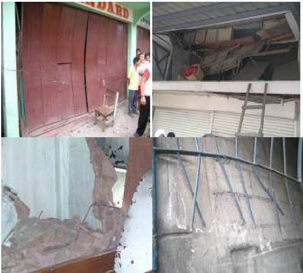
Figure 4: Other business establishment affected by the blast
