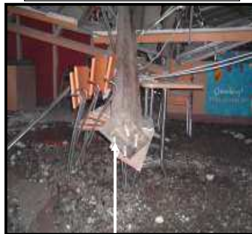
Detached steel beam cause by downward pressure
