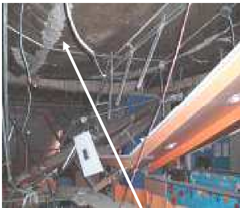
Crack concrete ceiling cause by strong pressure
