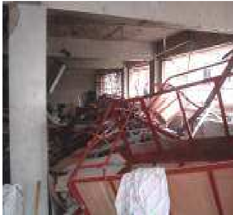
Debris at the second floor
