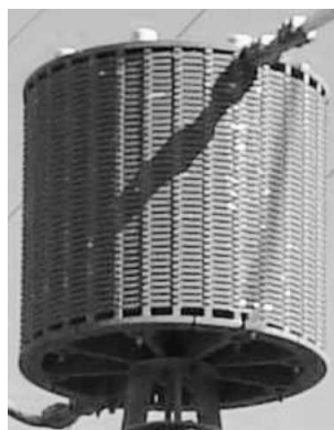
Figure 23 – HV line trap
