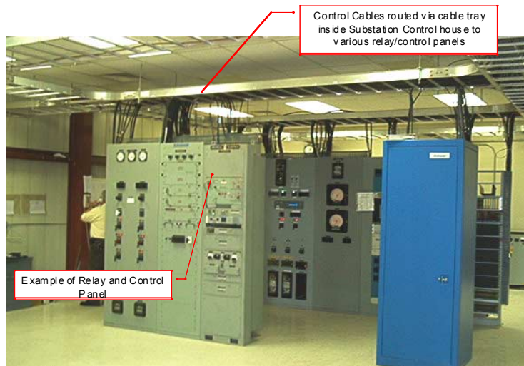
Figure 8 – Control cable access to equipment
