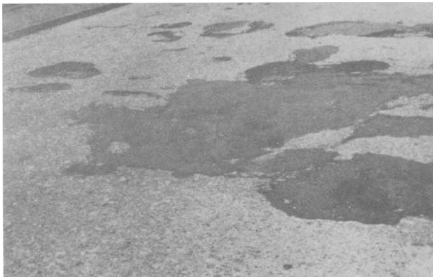
FIG. 1— Potholes (some patched) on a concrete bridge deck.
