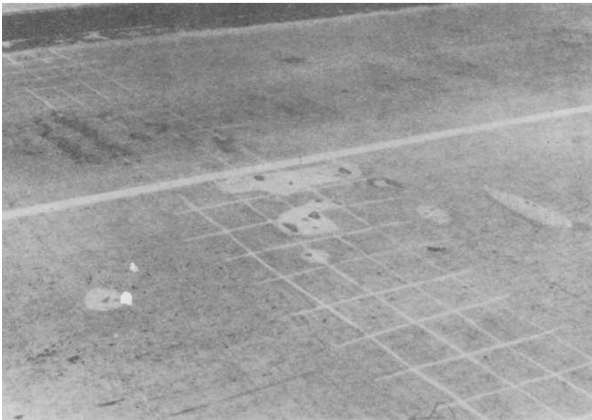
FIG. 2— Fracture planes and spalls. Extent of the fracture planes and the locations of the reinforcing bars are indicated.
