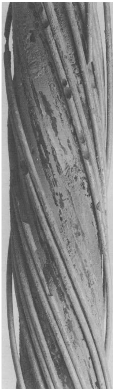
FIG. 1—Corrosion failure of neutral wires.
