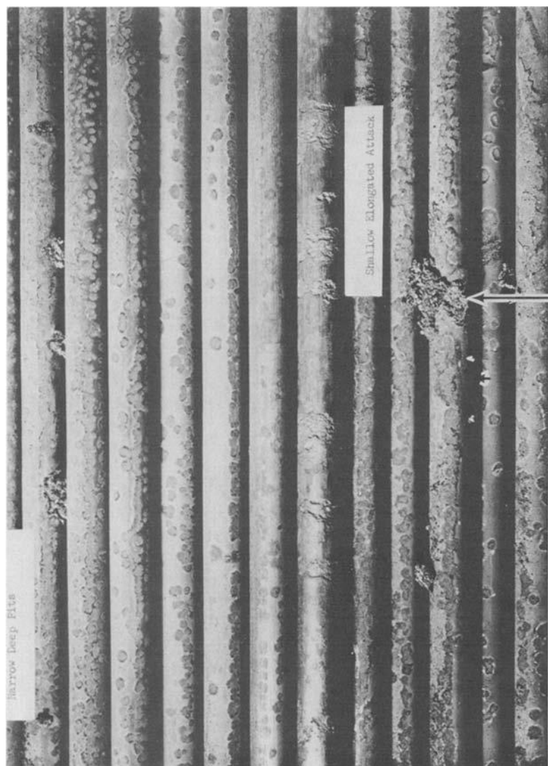
FIG. 4—Pitting attack, carbon steel heat exchanger tube. Note crystal-line appearance of corrosion products.
