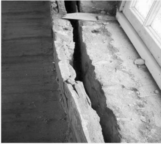
FIG. 20— Cement plaster at window sill level exhibits loss of adhesion, but not a loss of cohesive integrity.
