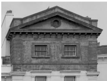
FIG. 1— Facade dating from the middle of the 19th century with stucco of dark-brown Harwich Roman cement; Harwich, England.
