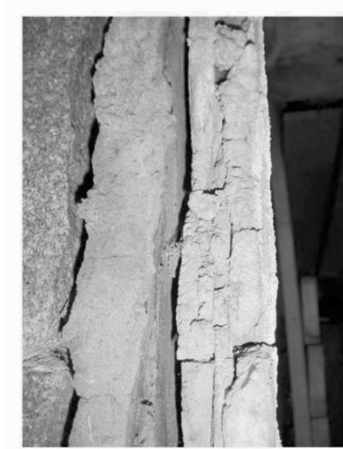
FIG. 21— Close-up view of cement plaster at the right side of the window, showing six distinct layers of cement plaster.
