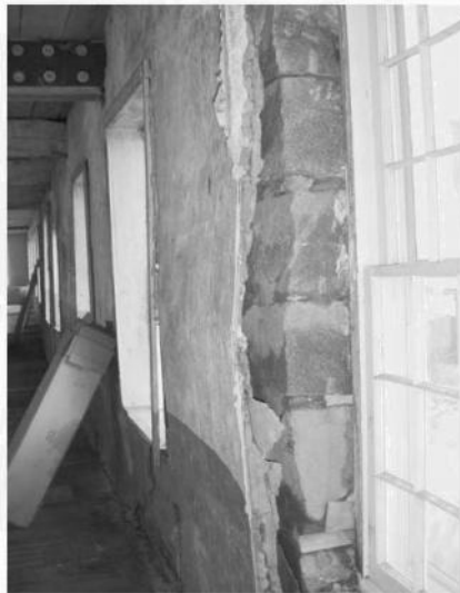
FIG. 18— Failing section of interior wall plaster.
