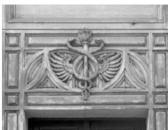
FIG. 3— Doorway lintel on a building dating from 1904–1906, Roman cement cast, showing the excellent state of preservation characteristic of this material; Cracow, Poland. The building has meanwhile been restored with the use of modern Roman cements.
