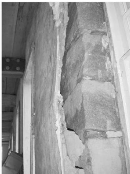
FIG. 19—Despite extreme displacement caused by a failing window, natural cement plaster remained intact, illustrating its flexibility.
