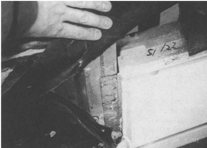
Figure 6 – Discontinuity of Casing Bead Flanges at a Window Head Corner
