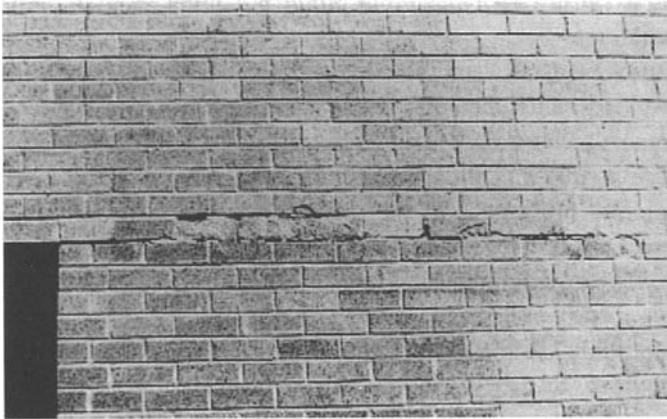
Figure 4 — Spalling of Brick Veneer at Shelf Angle Under High Compressive Stresses Due to Lack of Masonry Joint Under the Shelf Angle (from Drysdale et al [7]).
