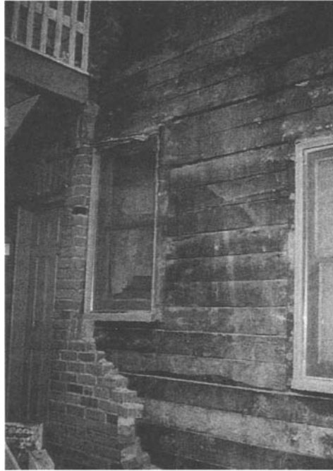
Figure 1— Masonry Veneer Damage at a Residential Building During Northridge Earthquake (from EERI [2]).
