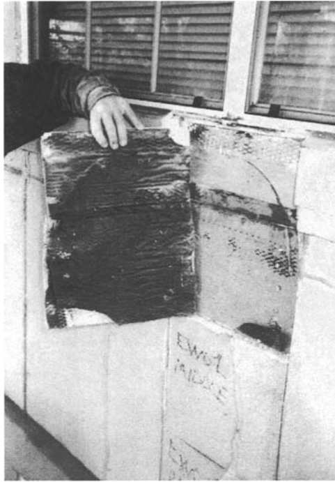
Figure 10 – Building Paper is Often Mis-shingled to Window Nailing Flanges
