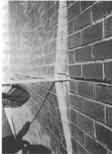
Figure 5— Buckling of Brick Veneer Wall Due to Vertical Differential Movement between Veneer and Frame (from Drysdale et al [7]).
