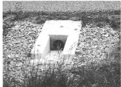
Figure 13 - Headwall and outlet for edge drain collector system.
