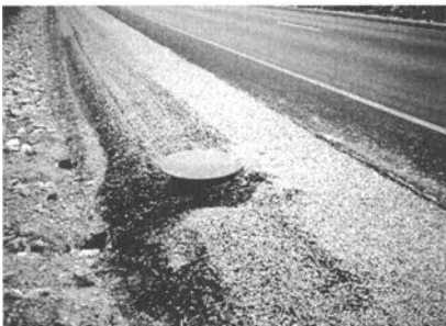
Figure 12 - View of temporary cover for top of edge drain collector and inspection port.
