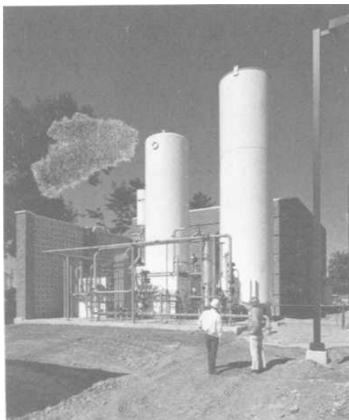
FIG. 1—High-volume oxygen users buy the gas in bulk, storing it in an adjacent facility.
