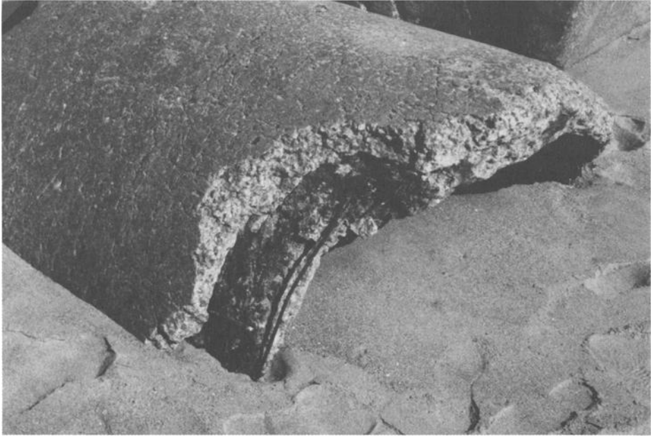
FIG. 10—Corrosion on reinforced concrete drain pipe on beach in Ventura, California.
