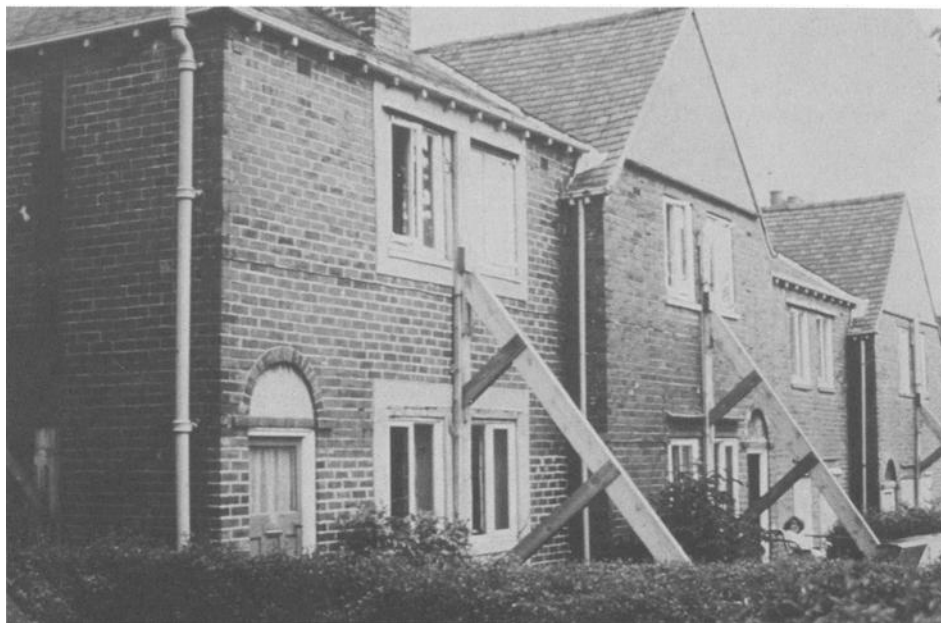
FIG. 4— Collapse of masonry walls due to corroded wall ties.
