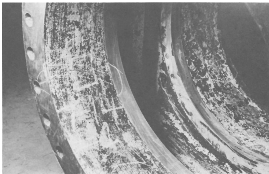
FIG. 3—Crack propagated to the interior surface on a 30-in. valve.
