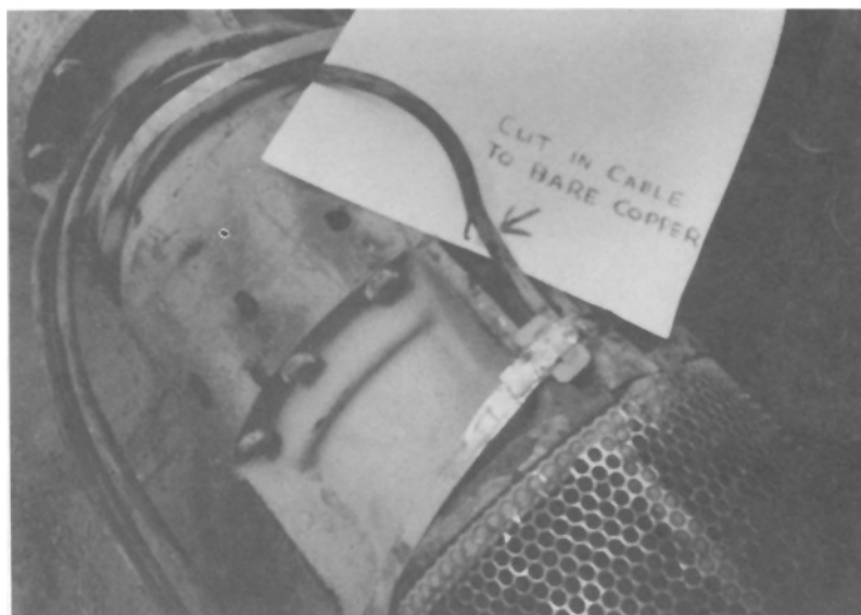
FIG. 17—Multiple perforations in the cast iron casing of a submersible pump. Damaged cable insulation led to stray current corrosion.
