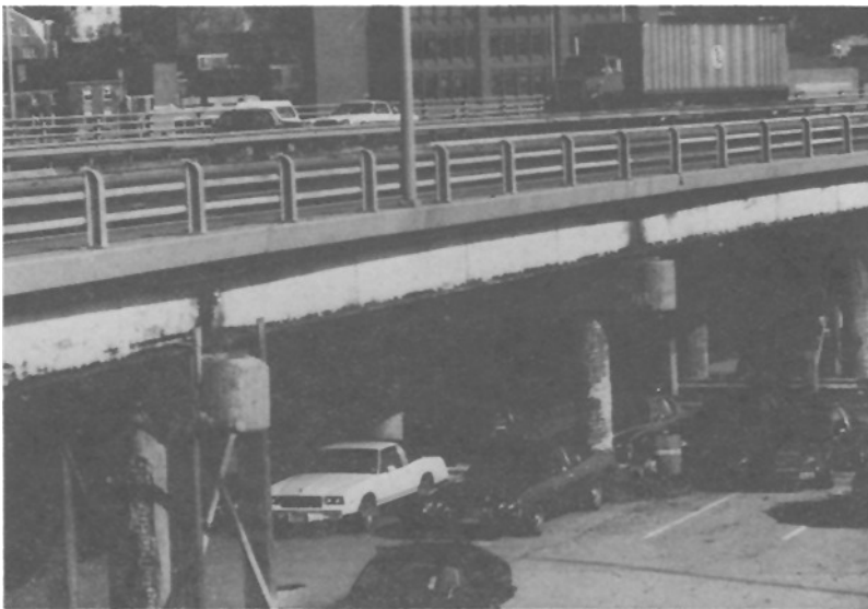
FIG. 2—Reinforcing steel corrosion causes spalling of concrete, making wood joists necessary for additional support on this elevated highway, Providence, RI.
