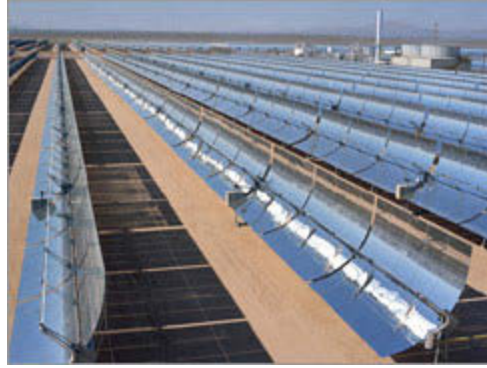
Figure 2 - Parabolic Trough Collector [2]
