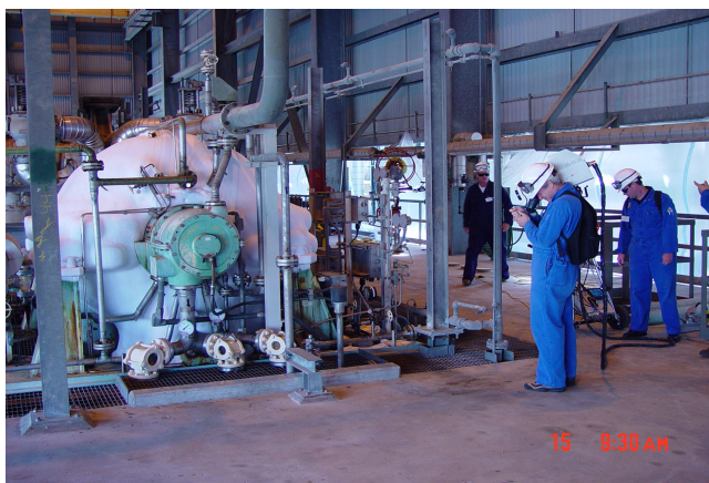
Figure ES 4-5. Scanning an Iced-over Compressor with CO 2 Laser at Ethylene Plant
