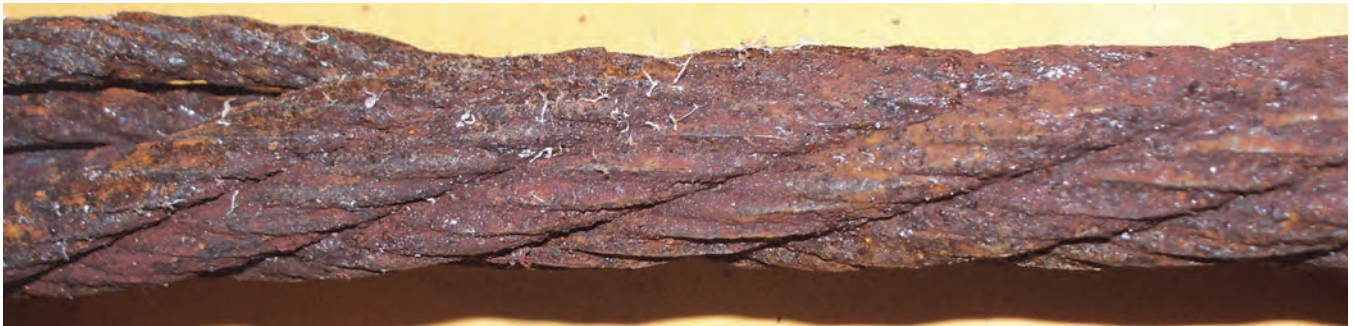
Figure 22—Example of Pitting Corrosion on a Wire Rope
