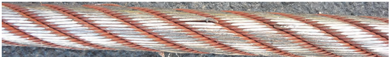
Figure 23—Example of Fretting Corrosion in a Wire Rope
