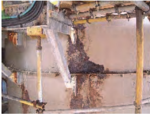
Figure 21—Example of a Design/Layout That is Difficult to Insulate
