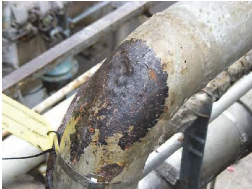
Figure 2—Jacketed piping with missing insulation plug (top photo) allowing water ingress and subsequently corrosion on piping elbow (bottom photo).
