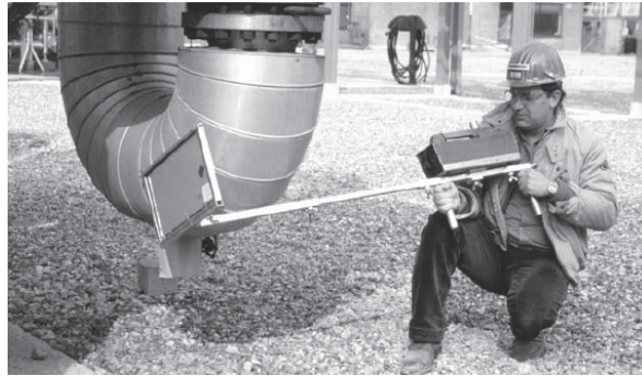
Figure 11—Photo of a Flash Radiography System for Pipe Profiling to Detect Wall Thinning Due to Corrosion
