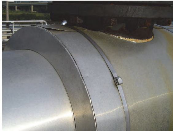
Figure 28—Example of Jacketing Joint with Missing Caulking
