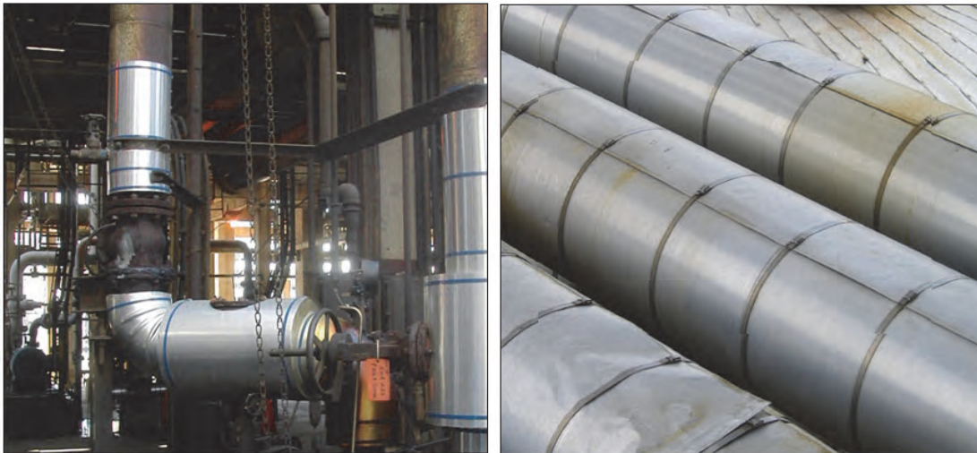
Figure 30—Examples of Joints with Poor Ability to Shed Water
