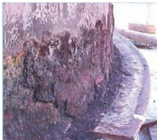
Figure 4—CUI at an Insulation Support Ring
