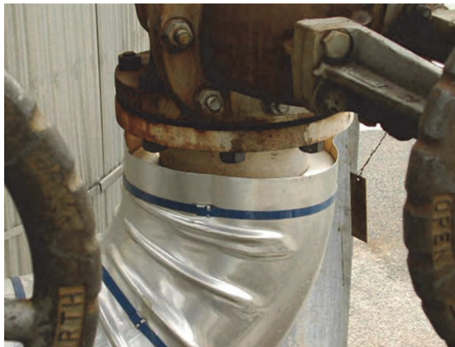
Figure 31—Example of Missing End Cap
