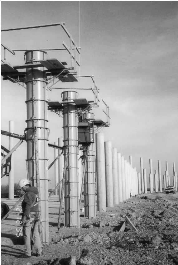
Round forms for grandstand support columns at The Texas Motor Speedway, Fort Worth, Texas. (Courtesy of EFCO Corp.)
