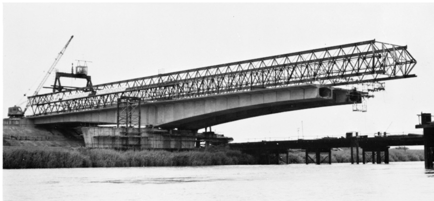
Prestressed concrete segmental bridge over the River Trent near Scunthorpe, Lincolnshire, England. (Courtesy of Cement and Concrete Association.)
