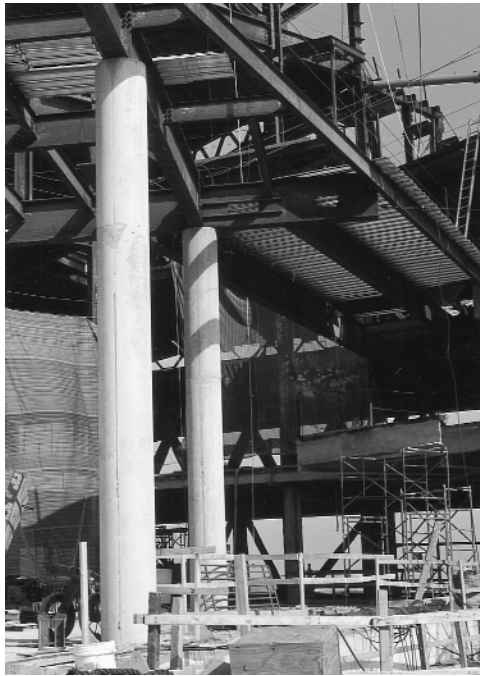
Reinforced concrete columns. (Courtesy of RSM Advertising, representing Molded Fiber Glass Products Company.)
