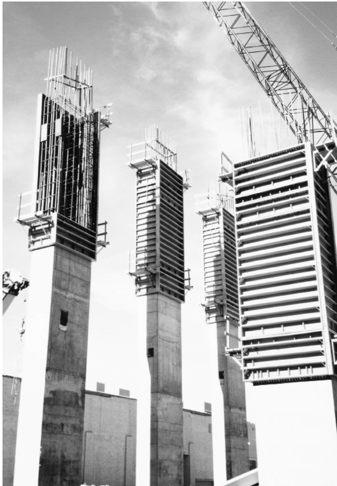
Richmond Convention Center, Richmond, Virginia. Notice column size changes. (Courtesy of EFCO.)
