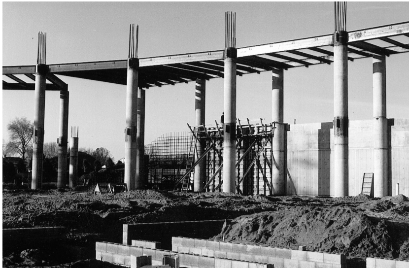
First Assembly Church in Wyoming, MI. (Courtesy of Veneklasen Concrete Construction Co.)
