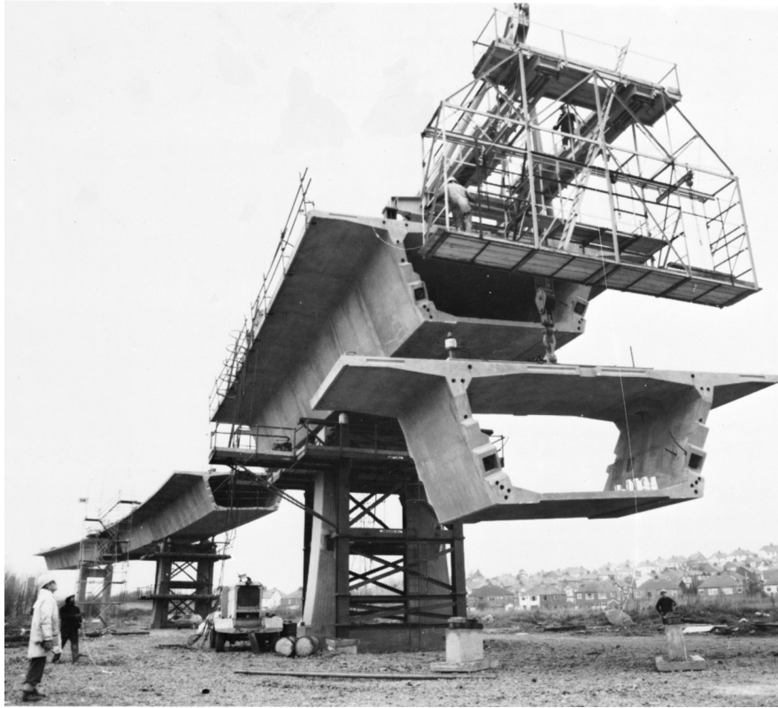
Posttensioned segmental precast concrete for East Moors Viaduct, Lanbury Way, Cardiff, South Wales. (Courtesy of Cement and Concrete Association.)
