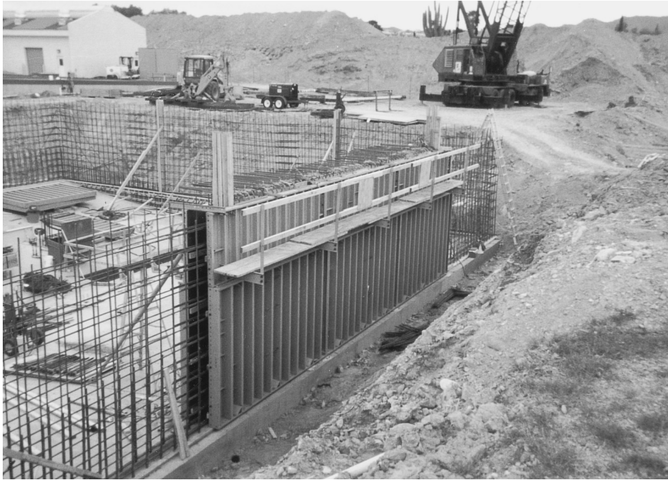
Fountain Hills, Arizona Wastewater Treatment Plant. (Courtesy of Economy Forms Corporation.)
