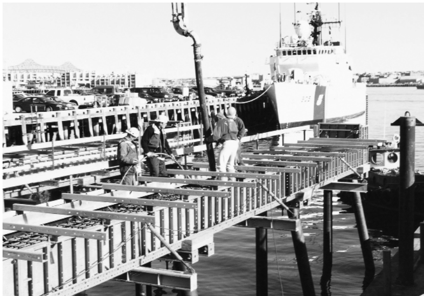
Finger piers for U.S. Coast Guard base, Boston. (Courtesy of EFCO Corp.)
