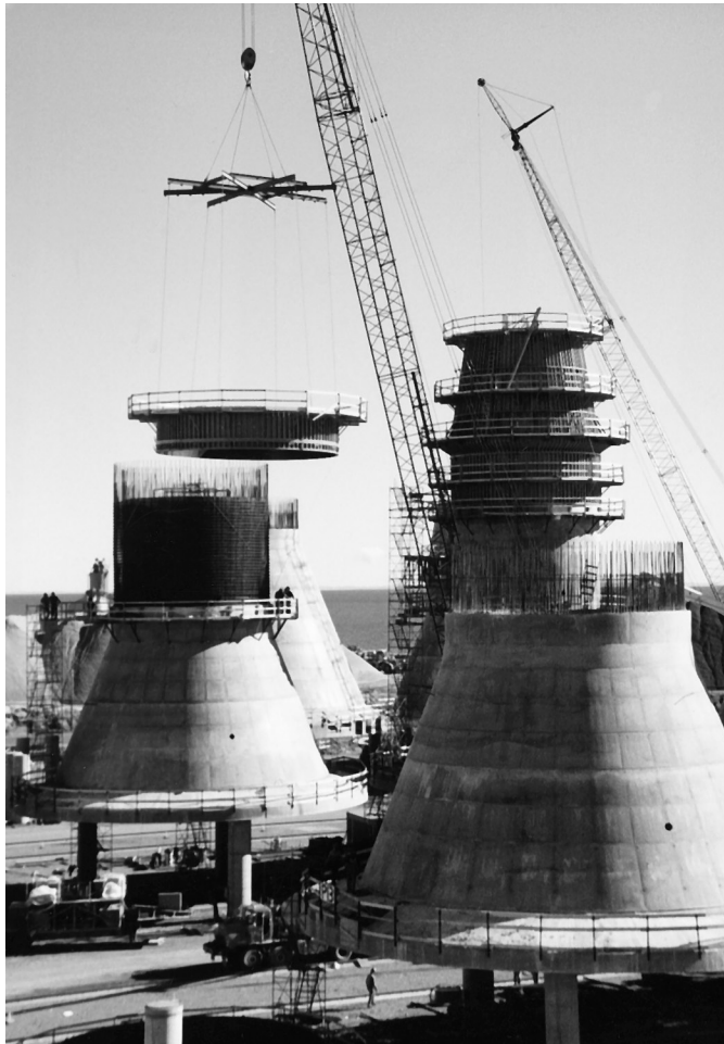
Pier bases for bridge from Prince Edward Island to mainland New Brunswick and Nova Scotia, Canada. (Courtesy of Economy Forms Corporation.)
