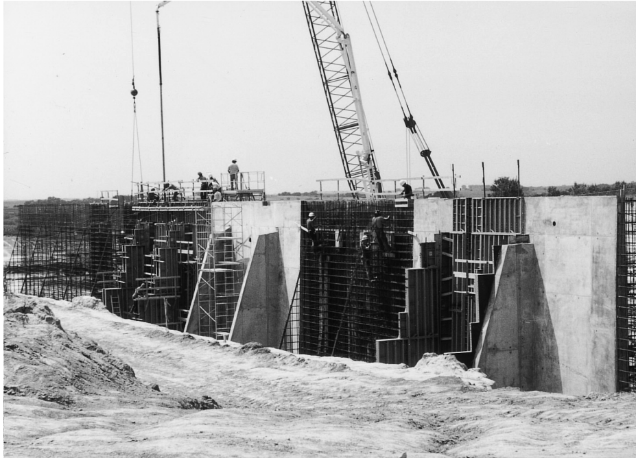
Thirty-two-foot-tall foundation walls for the MCI Mid-Continent Data Center in Omaha, Nebraska. (Courtesy of Economy Forms Corporation.)
