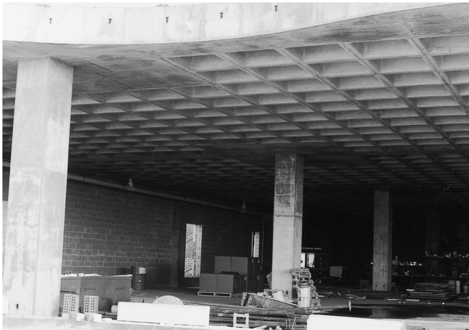
Cast-in-place concrete waffle slab, set with pan forms. (Courtesy of RSM Advertising representing Molded Fiber Glass Products Company.)
