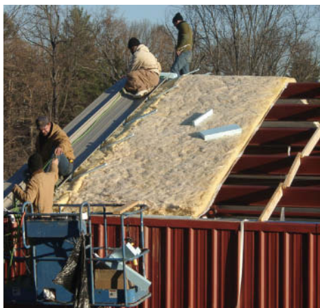
Fig. 7.3.7 The space between the sloped ceiling of this building and its actual roof is insulated with a thick mat of fiberglass insulation (left). The importance of that insulation is clearly visible on a snowy day, when the snow melts first where the fiberglass insulation is compressed by the beams and is therefore thinnest (right).
