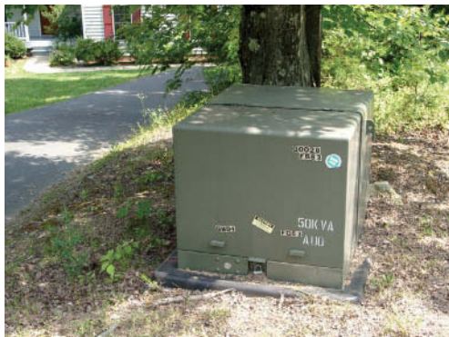
Fig. 11.2.13 This transformer transfers power from a medium-voltage underground circuit to a low-voltage underground circuit used by nearby homes. It handles 50 kV-A or 50,000 W of power.
