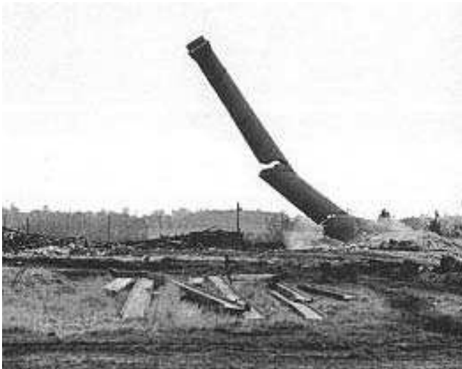
FIGURE 11.16 The 120 ft chimney of the former Co-op brush factory at Wymondham, Norfolk being demolished in 1988.
