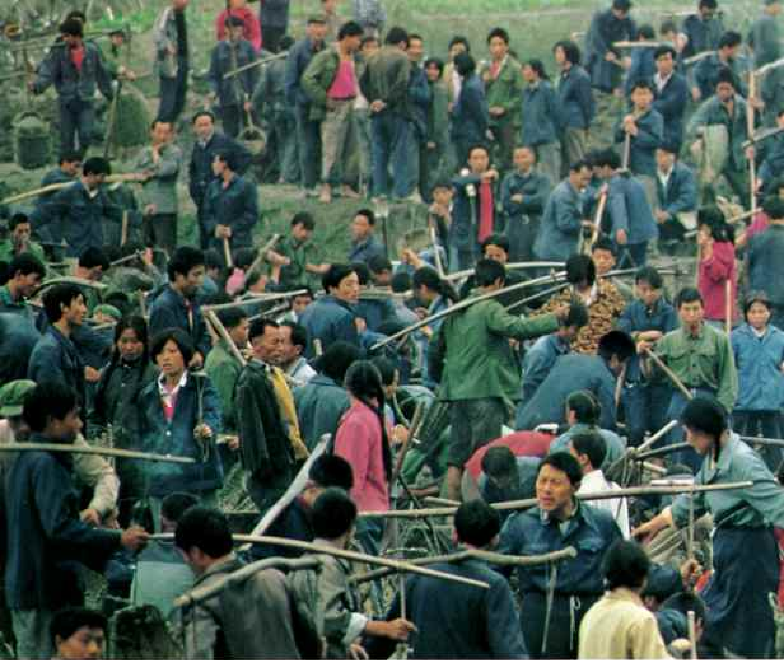
Pitching in on a gigantic scale at the request of the Central Committee, peasants who live along a 30-mile stretch of road between Chengdu and Guanxian widen
