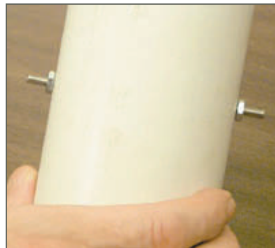
The installed positive electrode connectors
