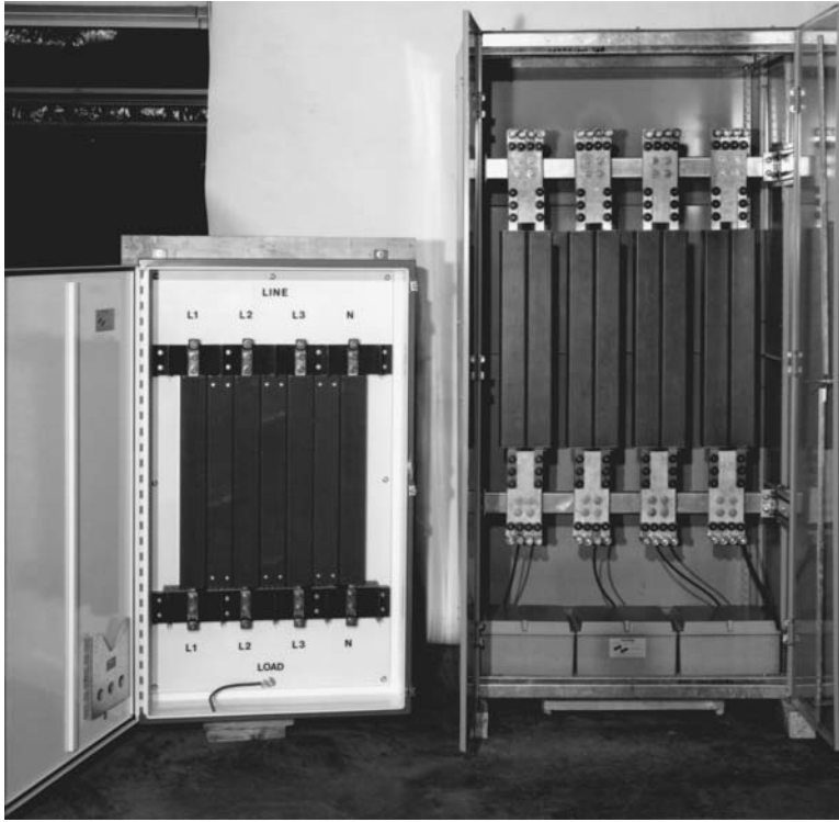
FIGURE 10.172 Interior view of a high-capacity hybrid power conditioner. (Courtesy of Control Concepts.)
