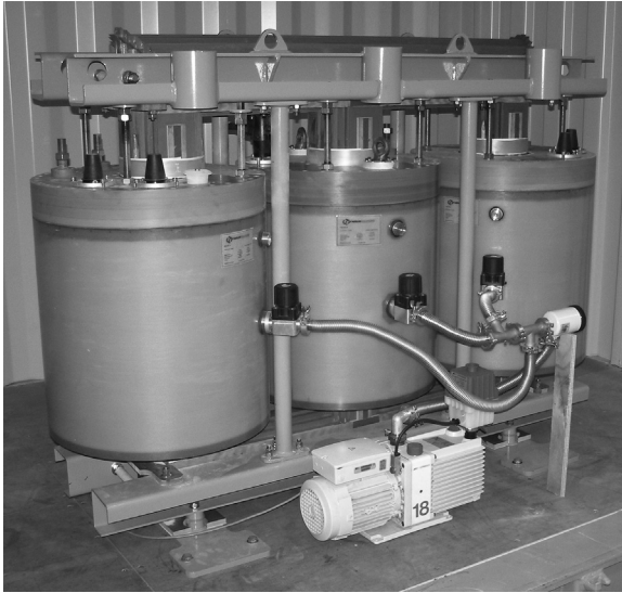
Figure 12.2 A 1 MVA 11/0.4 kV HTS transformer developed by a New Zealand/Australian team shown during assembly.
