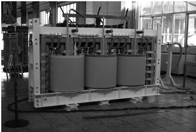
Figure 12.1 A 630 kVA HTS transformer developed by a Chinese team sponsored by the Chinese Academy of Sciences.
