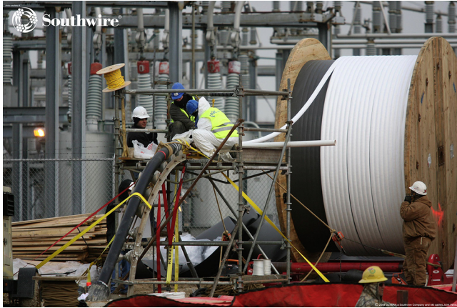
Figure 5.13 HTS Triax™ cable installation at the AEP Bixby substation. The white cable on the drum is the superconductor and dielectric portion being fed into the black cryostat and outer jacket of the final cable. The cryostat and outer jacket were already placed in a below-ground trench at the substation. The cable will be connected to the above-ground terminations in the background (Demko et al., 2007).
