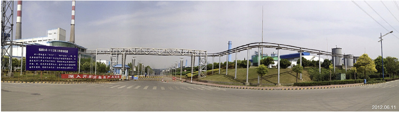
Figure 13.13 An overview of the 10 kA high-temperature superconducting DC power cable after installation.
