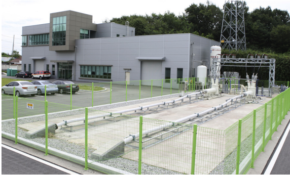
Figure 4.13 The Icheon substation on Korea is the site of a 410-m-long, 22.9-kV, 1.25-kA, 50 MVA 2G HTS-based cable installed by LS Cable using wire from AMSC. The cable is connected to KEPCO's grid. Courtesy LS Cable.
