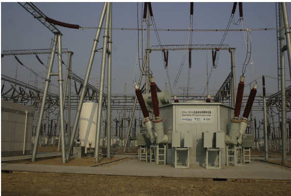
Figure 13.11 A view of the 220 kV/0.8 kA superconducting fault current limiters after installation at Shigezhuang substation in Tianjin.
