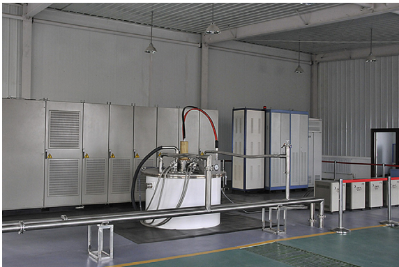
Figure 13.5 A view of the 1 MJ/500 kVA high-temperature superconducting magnetic energy storage.
