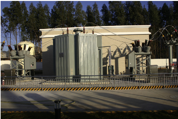
Figure 13.9 An overview of 35 kV/1.5 kA superconducting fault current limiters after installation at Puji substation.
