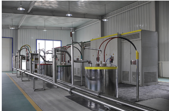
Figure 13.3 A view of the three-phase, 10 kV/1.5 kA high-temperature superconducting fault current limiter.
