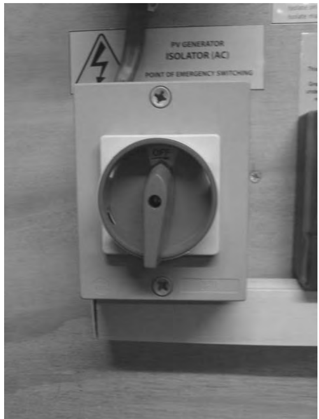
Figure 10-44 Solar DC isolator switch.
