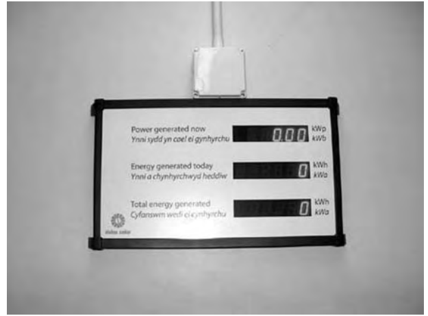
Figure 10-46 Awelamentawe school solar display. Image courtesy Dulas.
