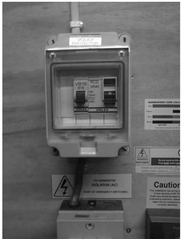
Figure 10-43 Mains circuit breaker.
