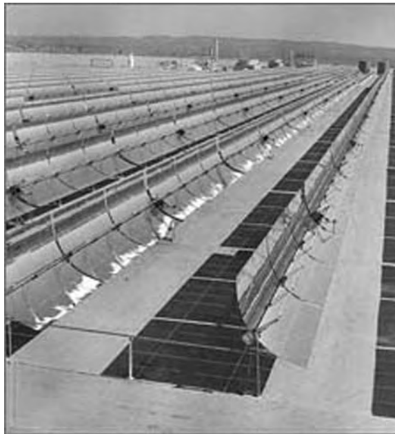
Figure 4-11 Solar thermal power in the Mojave desert. Courtesy Department of Energy.
