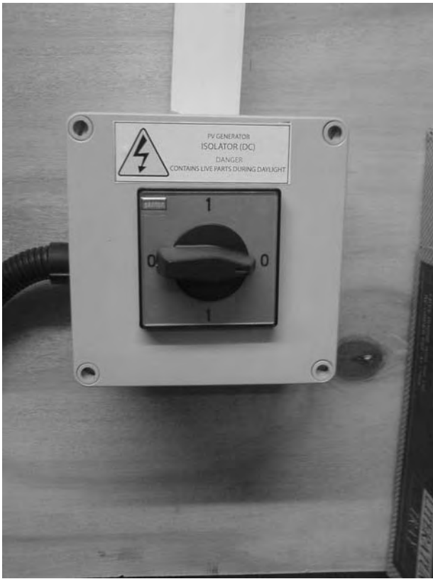
Figure 10-42 Mains isolator switch.
