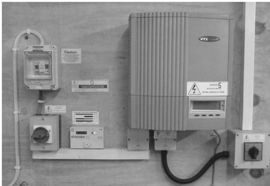
Figure 10-41 A typical inverter setup.
