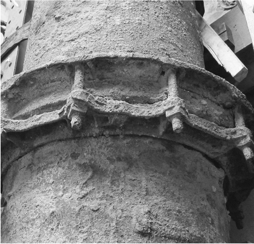
14.4 Externally corroded pipeline with flanged joint.
