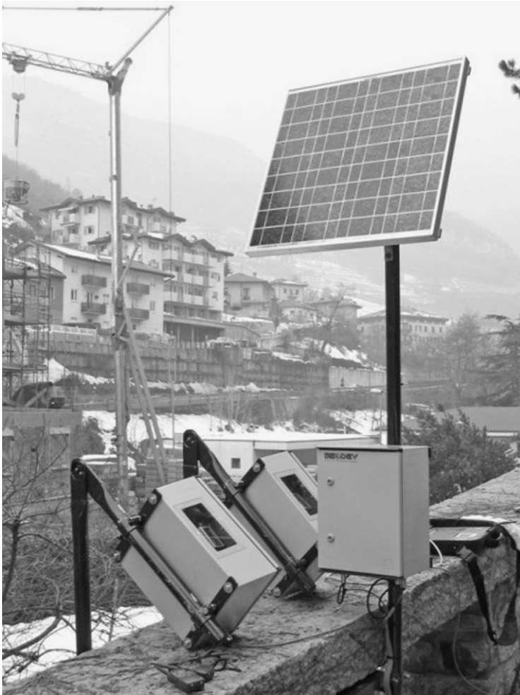
13.3 Laser distance meters, with protective housing, control system, and solar power supply. (Source: Picture courtesy SMARTEC SA.)
