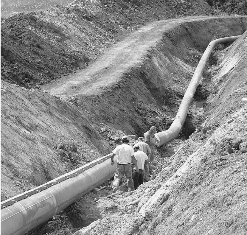
14.1 Continuous gas steel pipeline with welded joints (Glisic and Inaudi, 2007). (Source: Courtesy of SMARTEC.)
