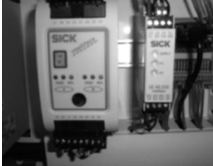
Figure 15-20 A safety controller on the left and a safety relay on the right.
