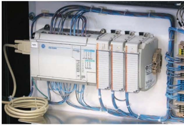
Figure 1-28 Single-ended PLC application. Source: Courtesy Rogers Machinery Company, Inc.
