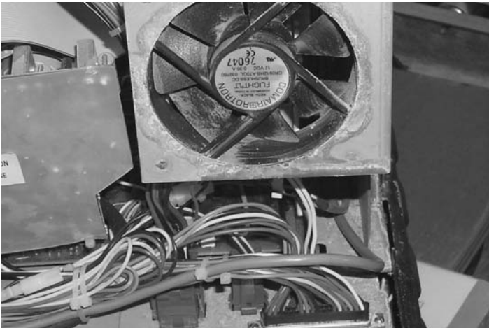
FIGURE 14.2 Corrosion of a fan bracket.
