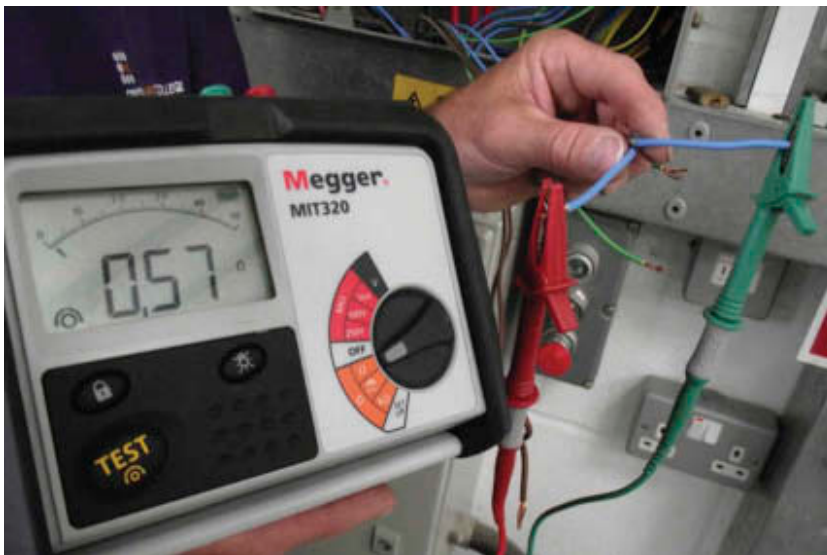
Figure 4.34 Test each end of the neutral conductor
