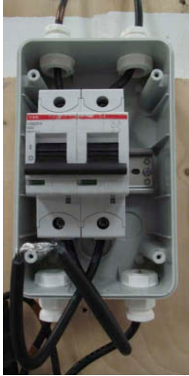
Figure 10.13 D.C. cables linked
