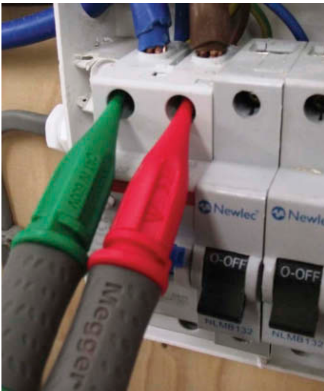
Figure 5.25 Test between incoming line and neutral
