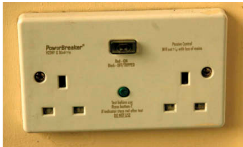
Figure 5.34 RCD socket outlet
