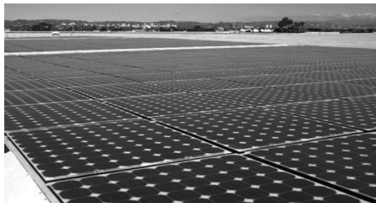
FIGURE 14.9 A rooftop PV system.
