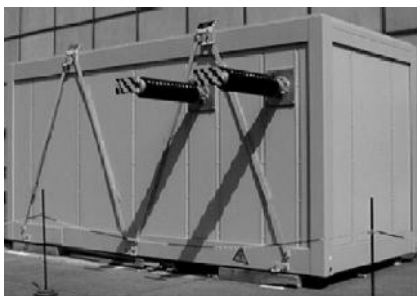
FIGURE 31.27 Compact outdoor container with an active dc filter.
