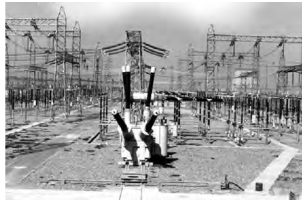
FIGURE 30.6 Spare converter transformer in the switchyard of an HVDC station.
