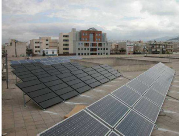
Fig. 5.8 PV roof mounted and grid connected
