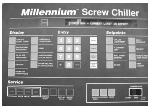
PLC control panel for chilled water supply
