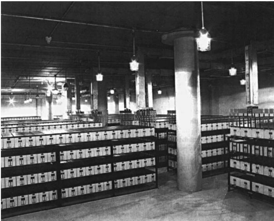
Fig. 12.26 Typical battery installation (courtesy of Invensys)
