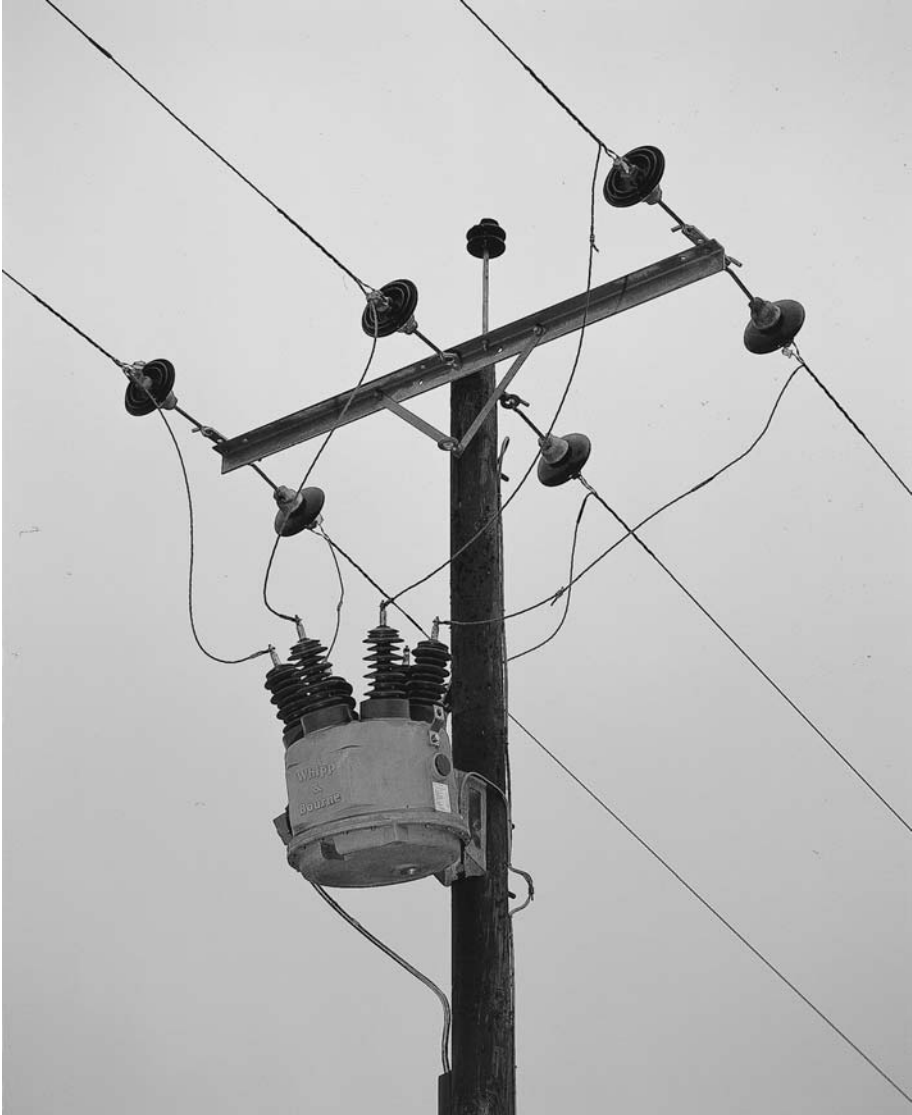
Fig. 7.20 11 kV pole-mounted auto-recloser (courtesy FKI plc – Engineering Group)
