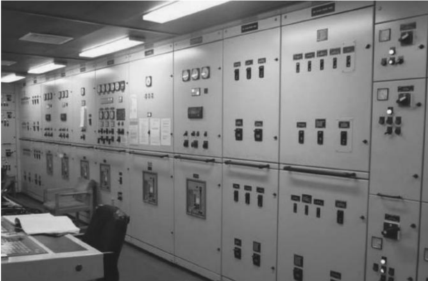
FIGURE 7.13 Typical main switchboard on large cargo ship. (From Raul Osigian, U.S. Merchant Marine Academy.)
