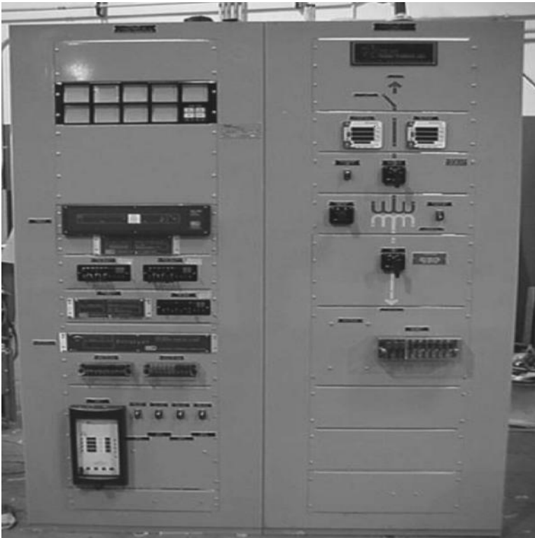
FIGURE 7.12 Generator switchgear (15 kV) in self-contained enclosure. (From Myers Power Products, Inc. With permission.)
