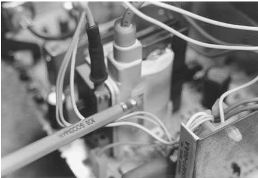
FIGURE 4-4 The high-voltage transformer found in a TV set.
