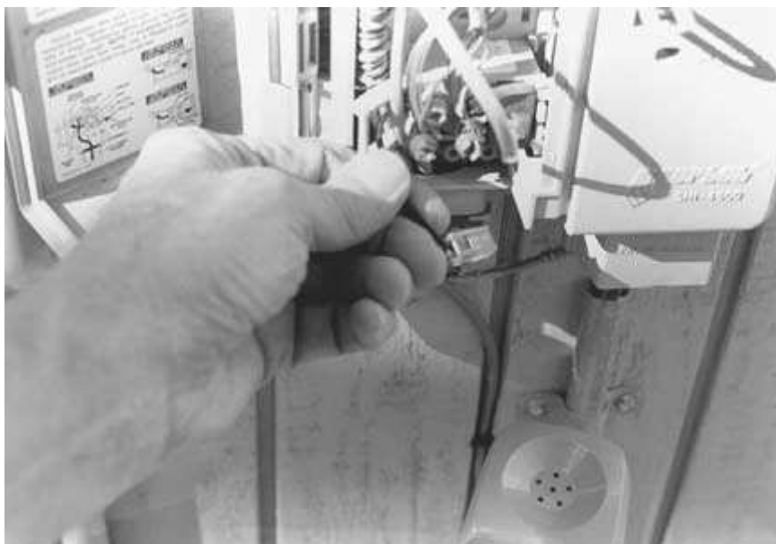
FIGURE 8-6 Modular plug being removed from the test box's interface jack.
