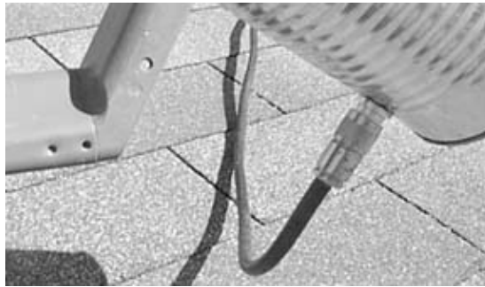
Figure 3-6. Dish antenna connector close-up
