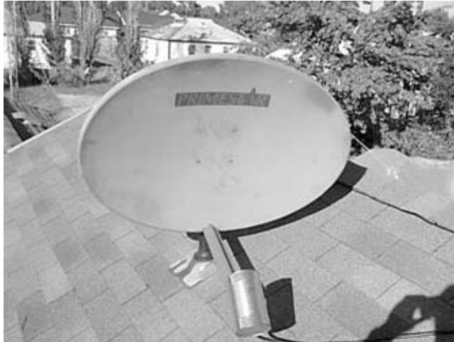
Figure 3-5. Mounted dish antenna
