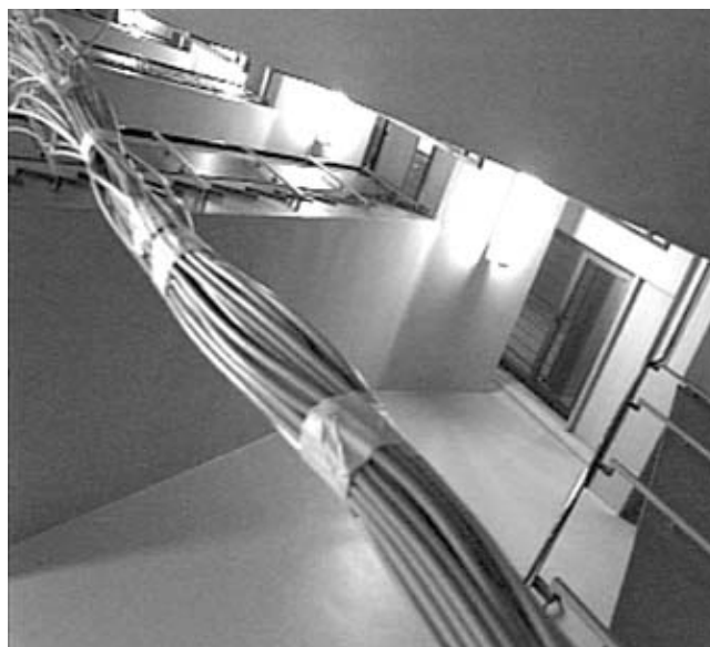
Figure 8-22. Cable bundles over cubicles
