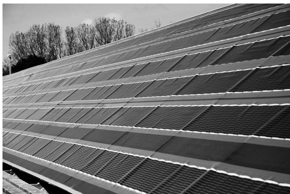
Figure 7.23 Solar park based on OPV, 250-square-metre wood panel with six solar-cell foils and an active area of 88 square metres.
