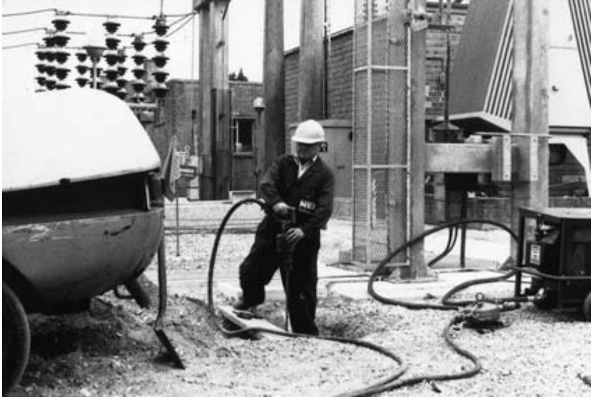
Fig. 7.11 Standard method showing copper-clad earth rod driven by a compressed air tool with compressor, as used by Stemet Earthing Co. Ltd.
