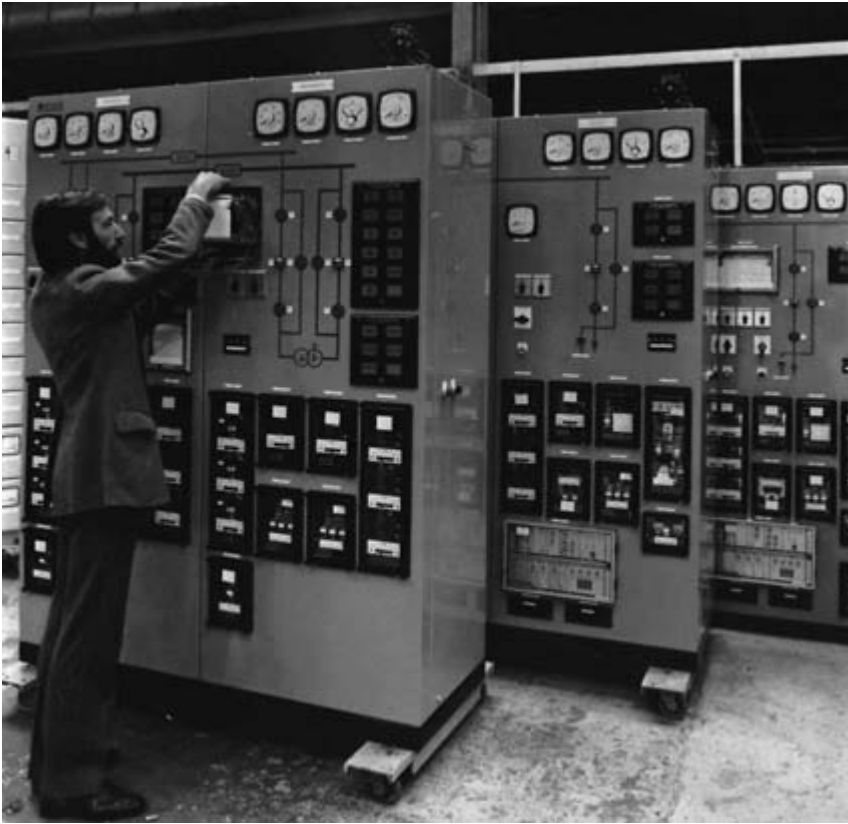
Fig. 2.11 Final adjustments being made on a control and instrumentation panel for Equador. Note the semaphores on the panel front ( Arcontrol Ltd ).
