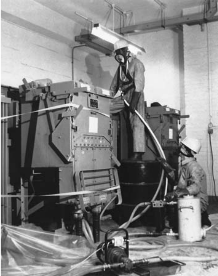
Fig. 13.3 Retrofilling of an askarel-filled unit in situ by R.F. Winder Ltd. The liquid is being replaced by silicone under carefully controlled conditions. Protective clothing is being worn by the operators.
