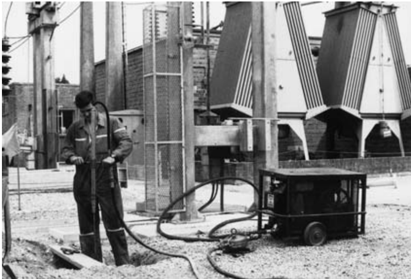
Fig. 7.10 New method showing a copper-weld earth rod driven by hydraulic 'mole' Grundomat ( T T. UK Ltd ).
