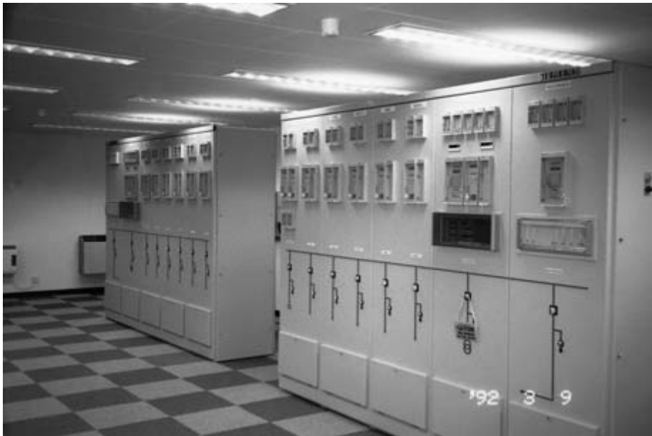
Fig. 2.2 Digital control panel, Jersey ( Siemens plc ).
