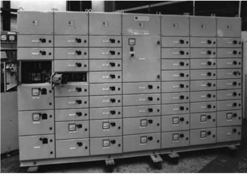
Fig. 2.13 The swing-out design on this l.v. motor control centre gives easy access to the components ( Arcontrol Ltd ).
