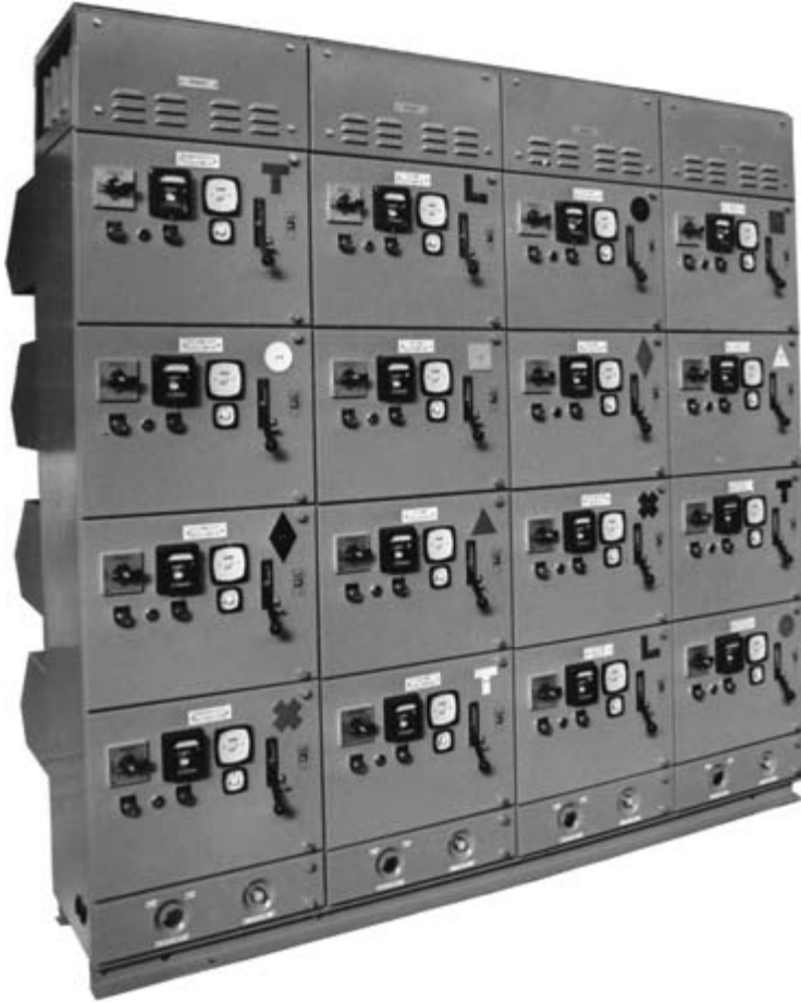
Fig. 2.12 A 400V power station distribution switchboard incorporating air circuit-breakers ( Electro-Mechanical Manufacturing Co. Ltd ).
