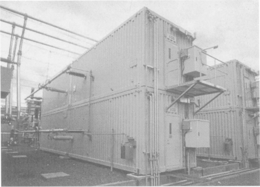
Figure 6-17: Thyristor Valves enclosed in containers at Garabi [ABB]
