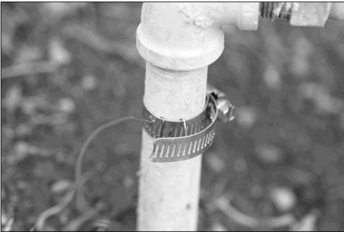
FIGURE 3-13: A good ground connection.
