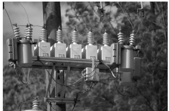
FIGURE 11-12 Capacitors used for power factor correction.
