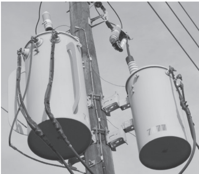
FIGURE 2-27 One transformer is larger than the other.
