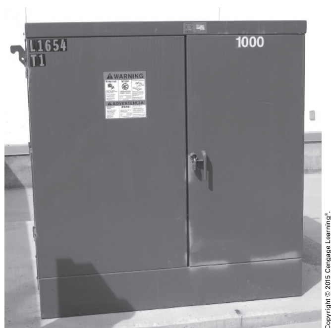
FIGURE 2-39 Pad-mounted transformers are generally contained in vaults.
