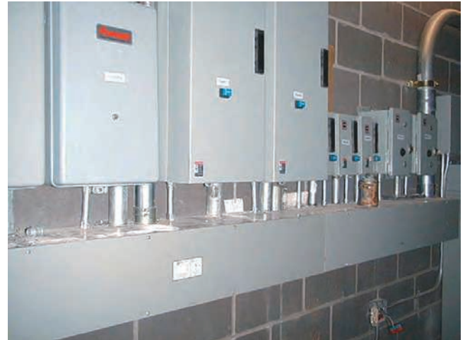
FIGURE 6-23 Wireway installed to facilitate wiring of motor disconnects and controllers.
