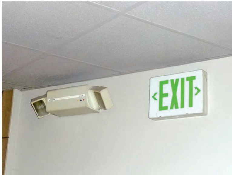
FIGURE 16-1 Unit equipment for pathway lighting and exit sign.
