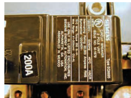
FIGURE 17-2 Circuit breaker is marked for 22 kAIR. Verify rating of panelboard assembly.
