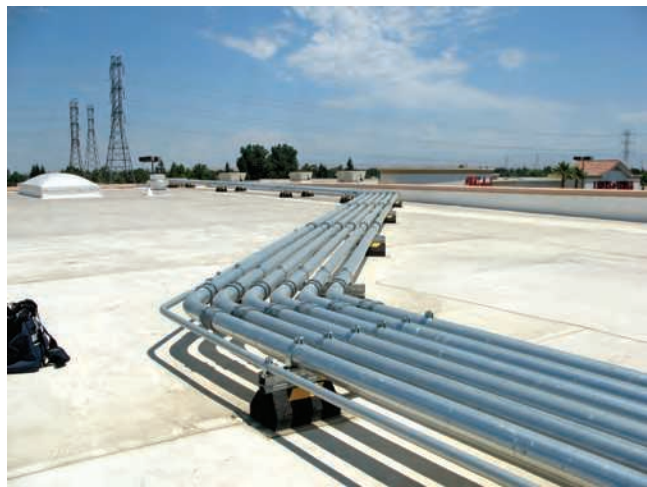
FIGURE 22-8 Commercial buildings often have conduit installations that are installed across a roof and are exposed to the rays of the sun.
