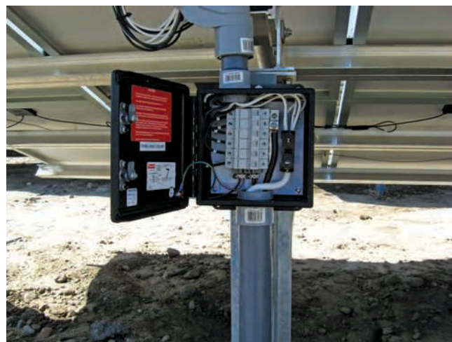
FIGURE 22-5 Fused combiner box.
