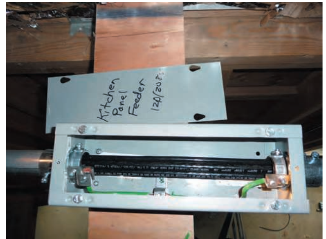
FIGURE 6-40 Straight-through pull not smaller than 8 times the largest trade size (metric designator) of the conduit or tubing.
