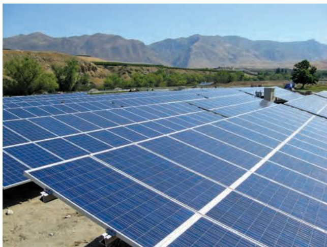
FIGURE 22-4 A ground-mounted array of modules.
