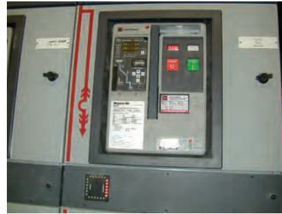
FIGURE 17-29 Circuit breaker with solid-state controls to shape tripping curve.
