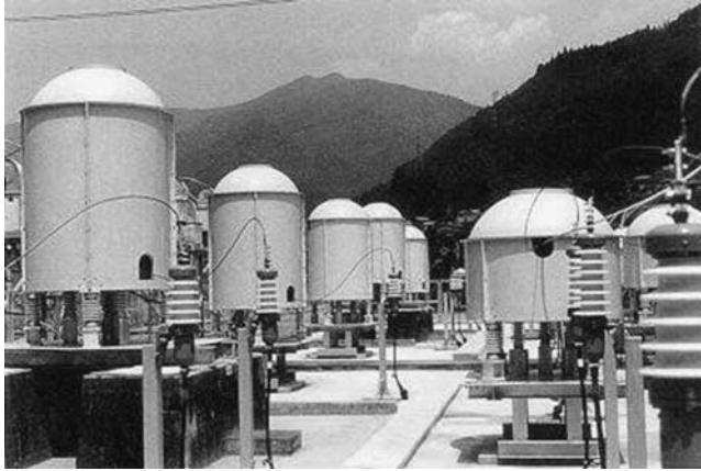
FIGURE 2.9.43 Installation of harmonic filter reactors for an HVDC project with a sound-shield enclosure.
