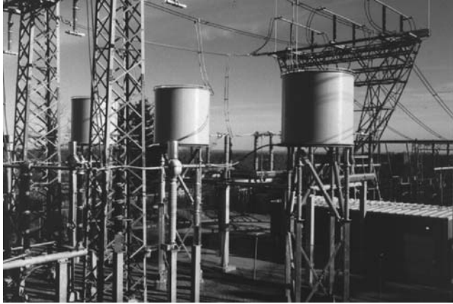
FIGURE 2.9.6 345-kV phase reactors.
