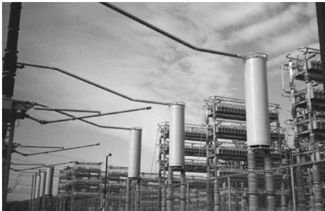
FIGURE 2.9.16 550-kV capacitor inrush/outrush reactors.
