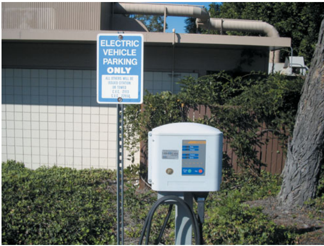
FIGURE 42-28 A typical electric vehicle charging station on the campus of a college in southern California.
