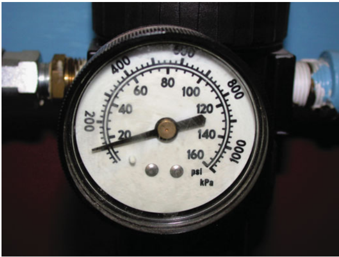
FIGURE 1-78 The air pressure going to the nozzle should be reduced to 30 PSI or less to help prevent personal injury.
