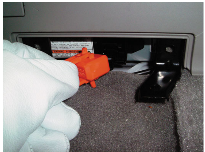
FIGURE 1-85 The high-voltage disconnect switch is in the trunk area on a Toyota Prius. High-voltage lineman's gloves should be worn when removing this plug. (Courtesy of Tony Martin)
