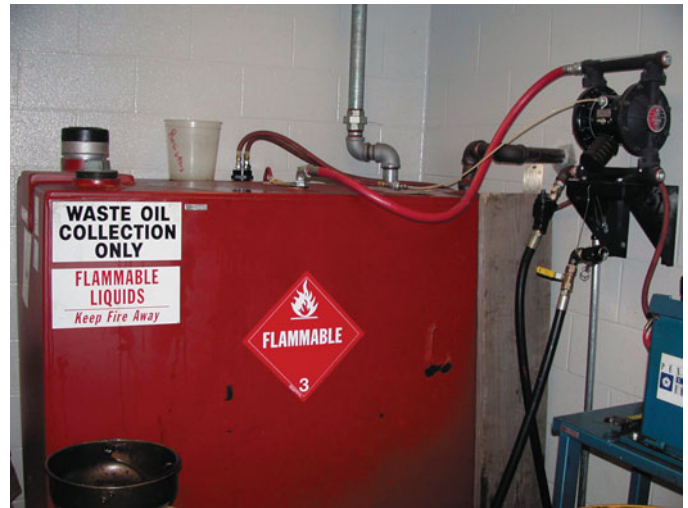
FIGURE 2-3 A typical aboveground oil storage tank.
