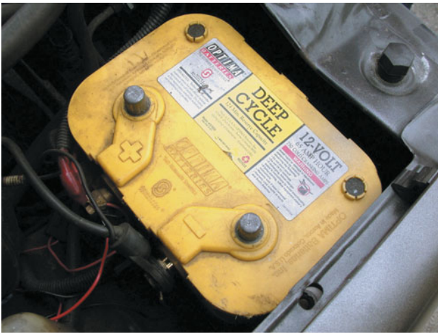
FIGURE 15-9 An absorbed glass mat battery is totally sealed and is more vibration resistant than conventional lead-acid batteries.
