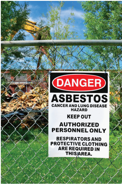
Figure 1.35 Hazardous areas should be clearly signposted.
