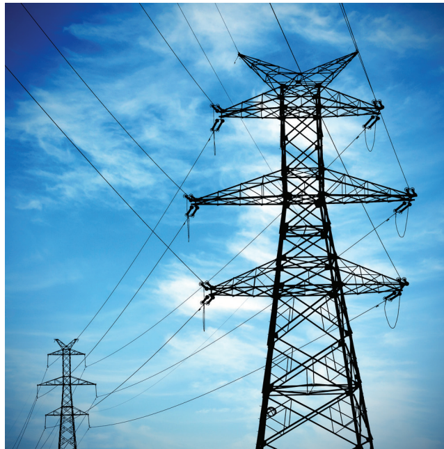
Figure 3.10 Transmission line steel pylon.
