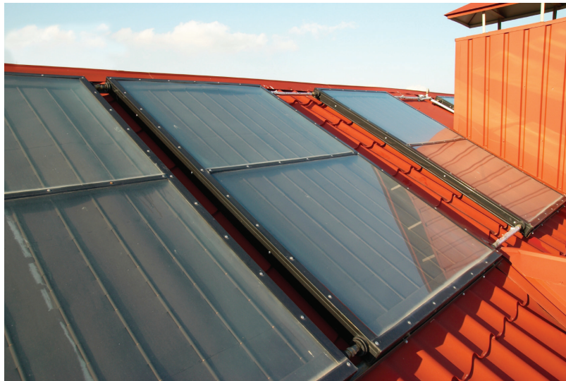
Figure 3.17 Solar hot water panel.
