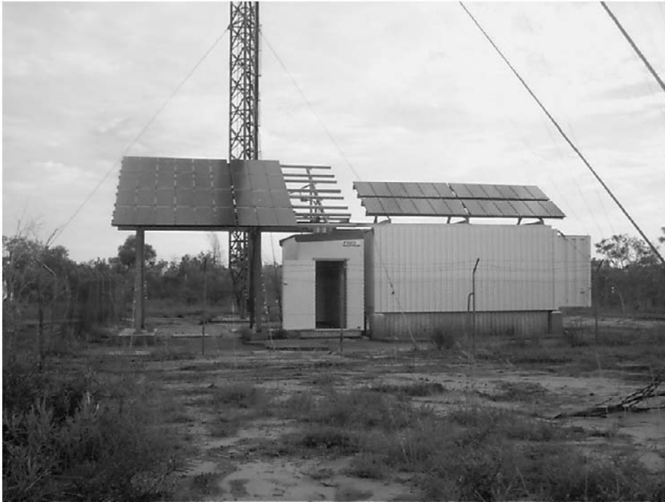
Figure 8.2. The first solar-powered mobile telephony base station in the Telstra network, located at Roebuck plains, Western Australia, (Used with permission of Silcar Pty Ltd. Design & Construction)
