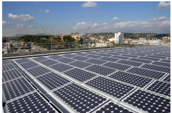
FIGURE SE2–4 Large array of solar panels. NREL.gov.
