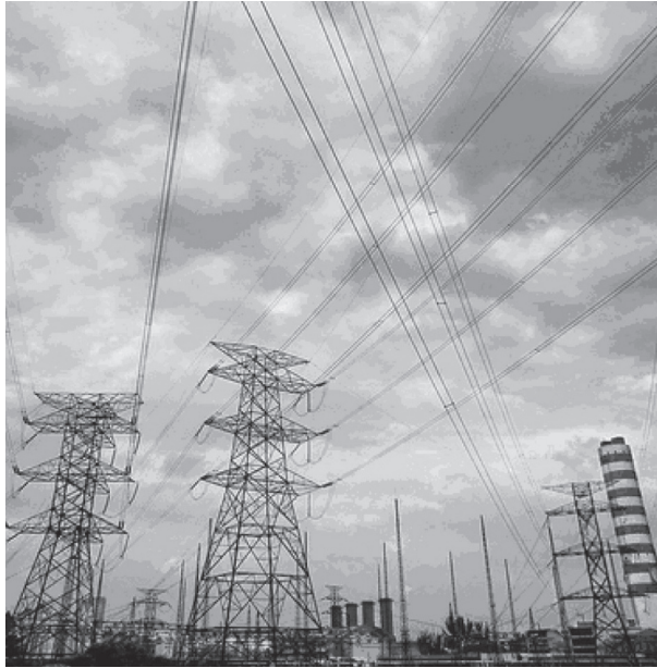
FIGURE 7.5 Transmission lines out of Connaught Bridge Power Station, Malaysia.
