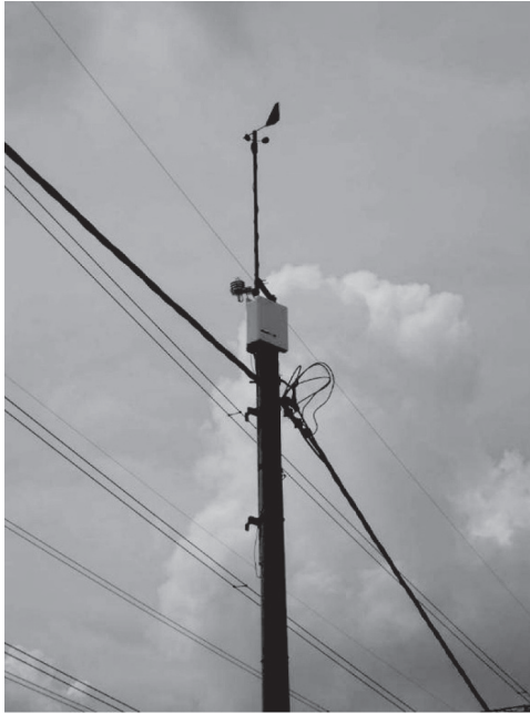
FIGURE 7.16 Weather monitoring using a weather station for transmission line in Malaysia.
